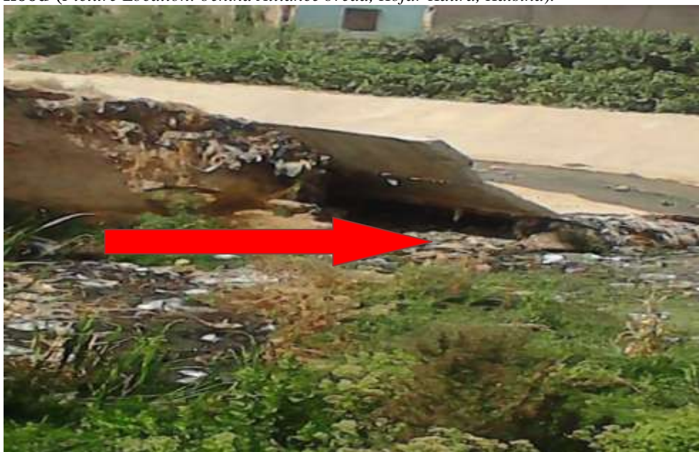
Plate 2: Damage to culverts by flood (Picture Location: Near Lambun Sarki, Kofar Marusa, Katsina).
