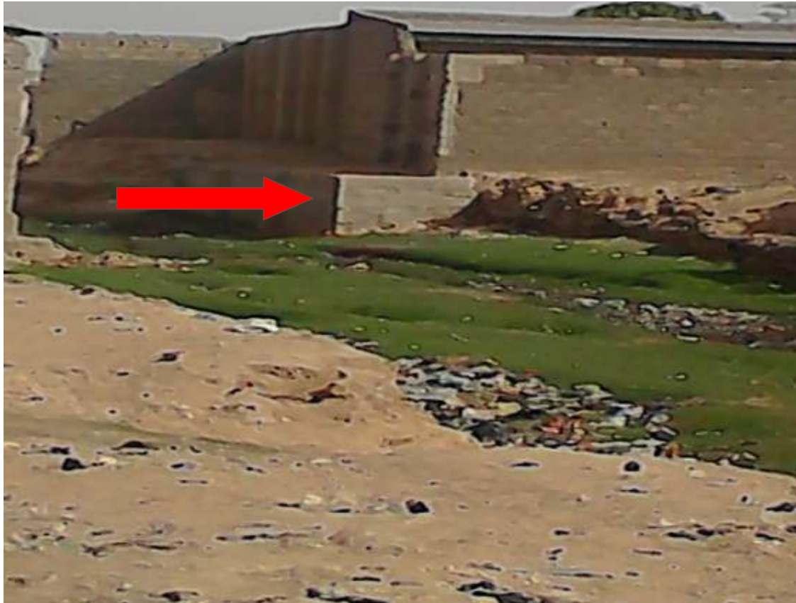
Plate 1: Construction of retaining wall/raising house up above flood level as a coping strategy to flood (Picture Location: behind Alliance bread, Kofar Kaura, Katsina).
